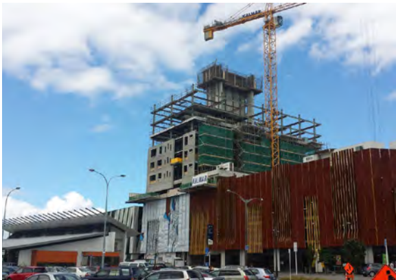
Construction of new carpark and Apartment building in New Lynn central. 2013. Image: http://transportblog.co.nz/wp-content/uploads/2013/11/New-Lynn-Apartment-construction-1.jpg .
